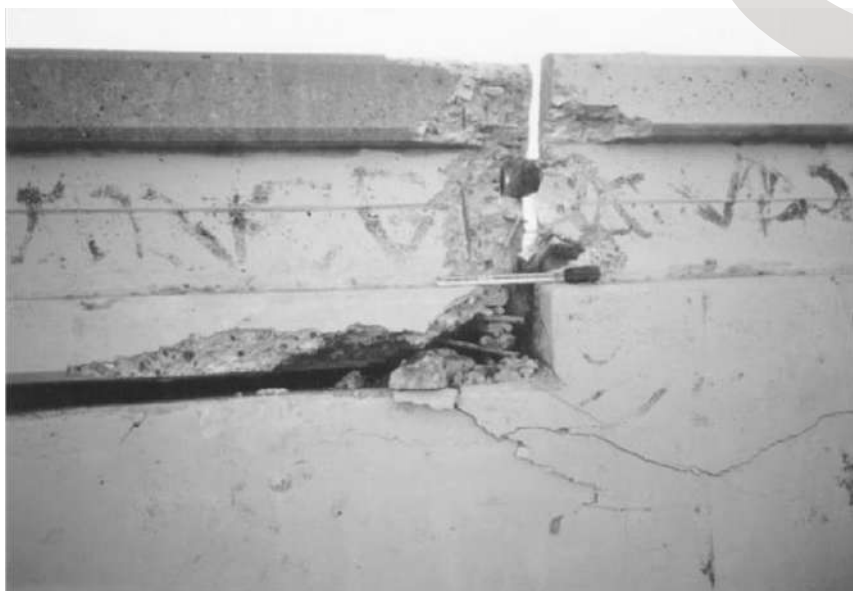
1.3 Santa Clara River Bridge pounding damage to the abutment in 1994 Northridge Earthquake (source: Chen and Duan [2000]).
