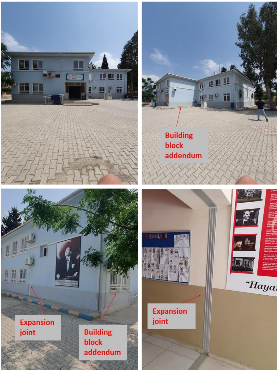
Fig. 7 – Photos that highlight the newly added building block next to the existing school structure (a, b, c) and location of expansion joint between new and existing structure (d).
