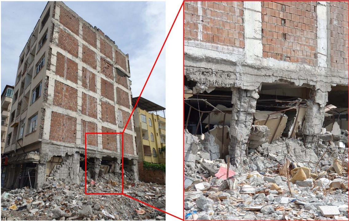
Fig. 6. Very severe damage on a r.c. building due to soft-storey mechanism.
