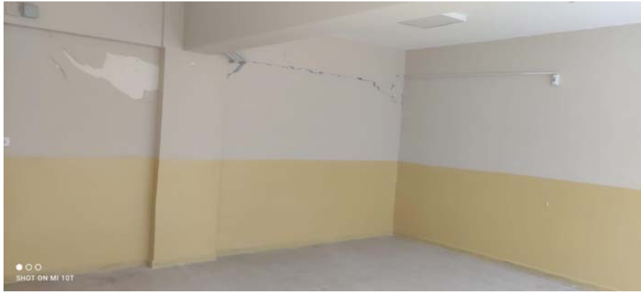
Fig. 4. Detachment at the interface between the original r.c. frame and the wall adopted as strengthening system.
