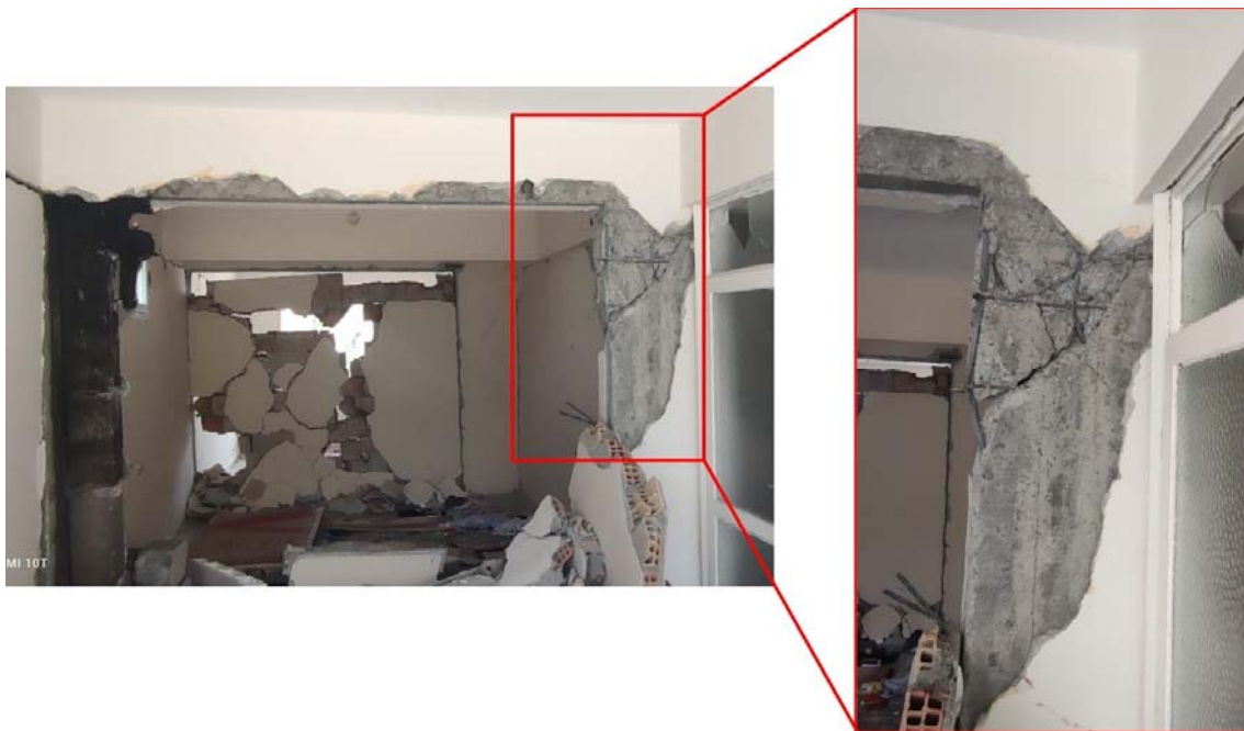
Fig. 5. Brittle shear failure of a r.c. column due to interaction with infills.
