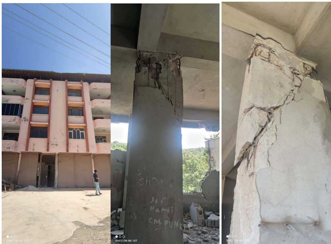
Fig. 19 Shear failure of several RC columns near the stairwells
