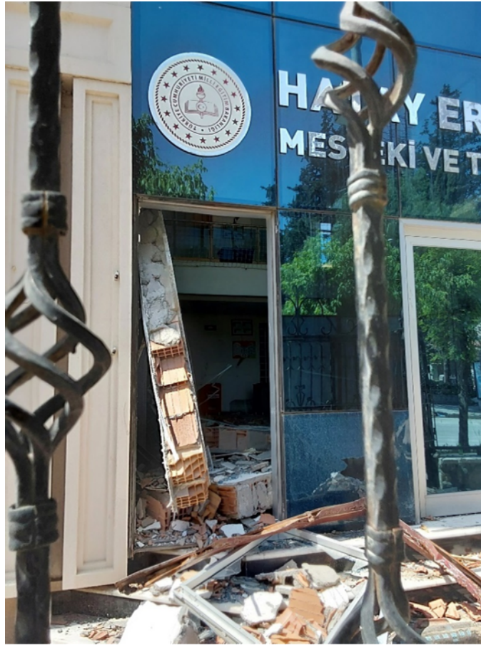
Fig. 12. Overturning of internal masonry separation walls
