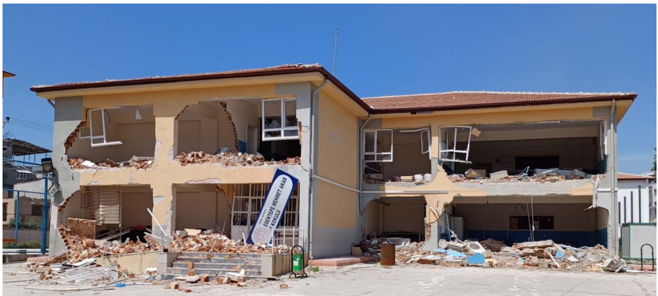
Fig. 11. Out of plane collapse of the infill walls on both floors.
