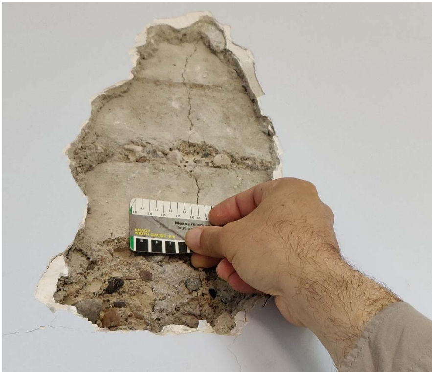
Fig. 3. - Position on a flexural crack on a beam.
