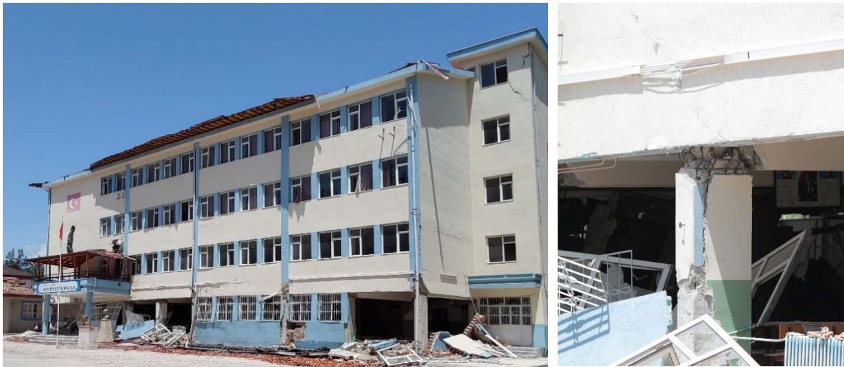
Fig. 9. Soft storey effect due to partial collapse of the front infill walls; plastic hinging of the columns.
