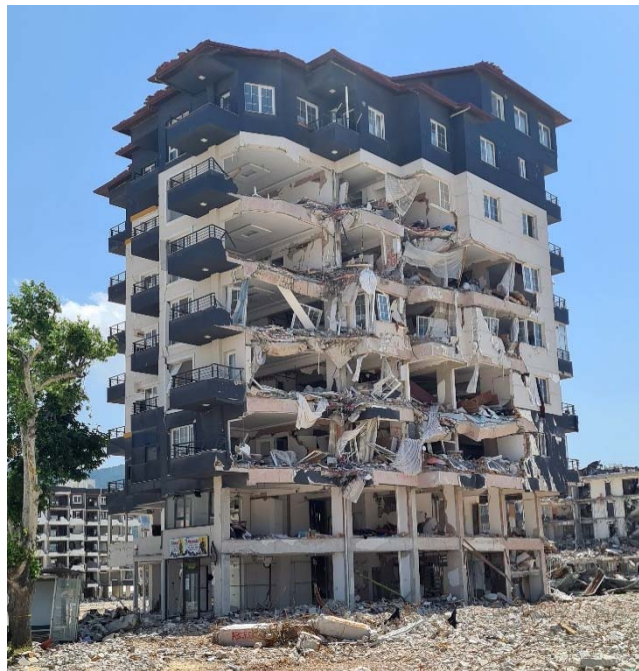
Fig. 18 Collapse of the external infill walls and damage to the perimeter beams lacking direct column support.
