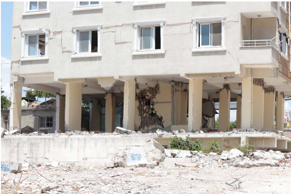
Fig. 16. Shear failure of an RC shear wall and plastic hinging at the top of the ground floor columns.
