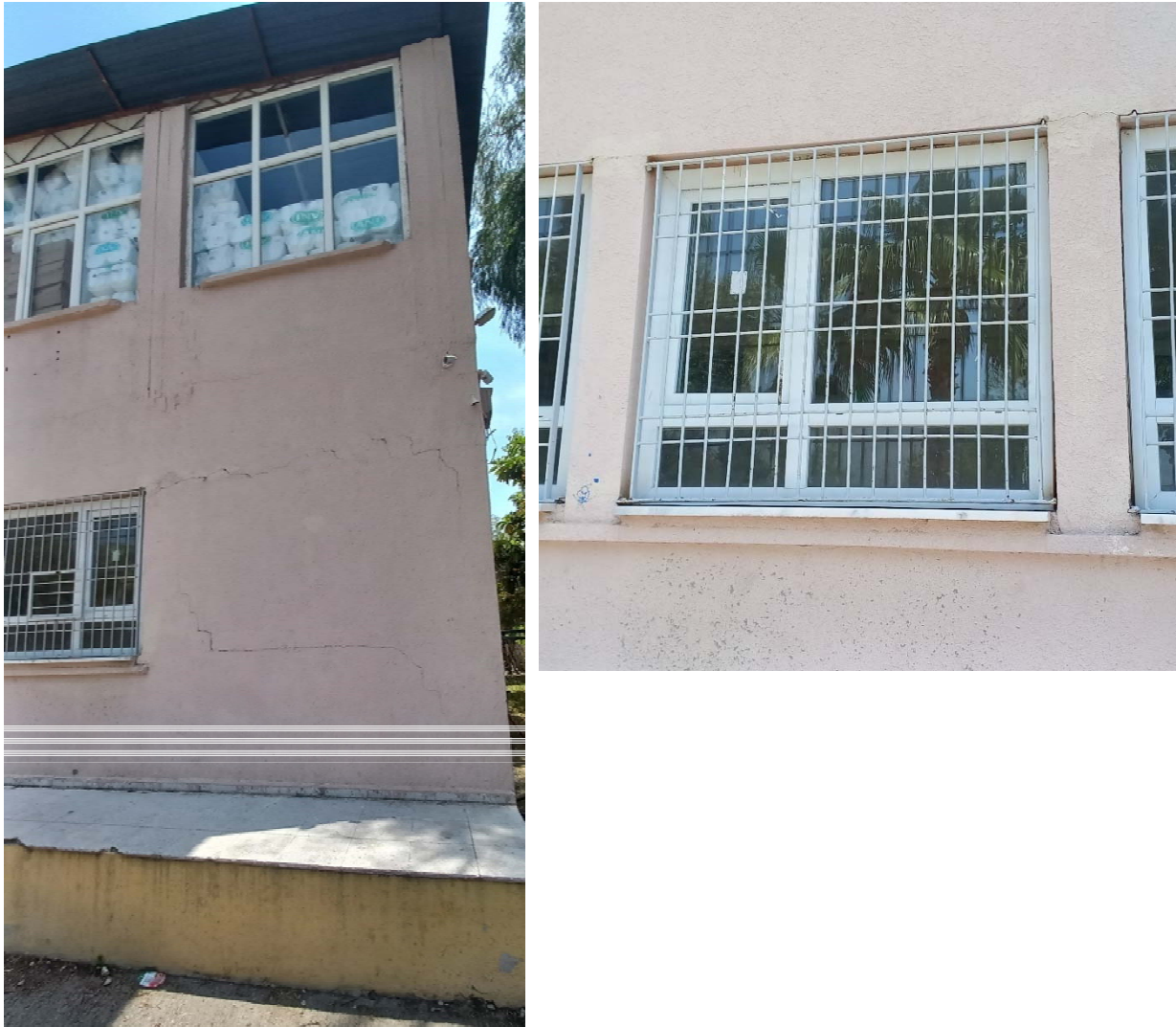
Fig. 13: Light damage at the interface of the infill walls
