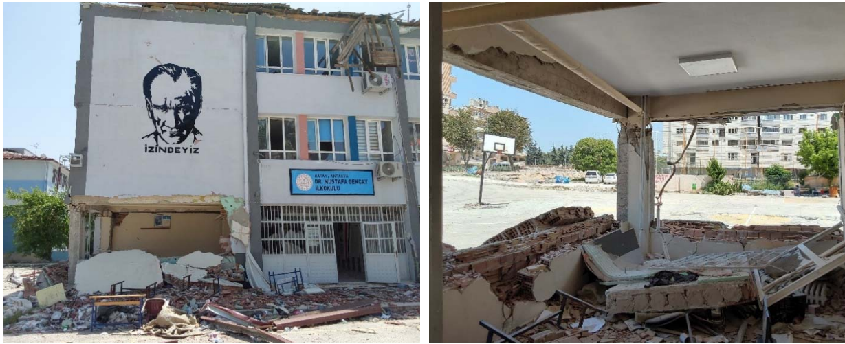
Fig. 8 Left panel: front view; right panel: view from the inside, collapsed external infill masonry walls and plastic hinging of the adjacent columns with clear disorganization of the concrete nucleus due to lack of adequate passive confinement
