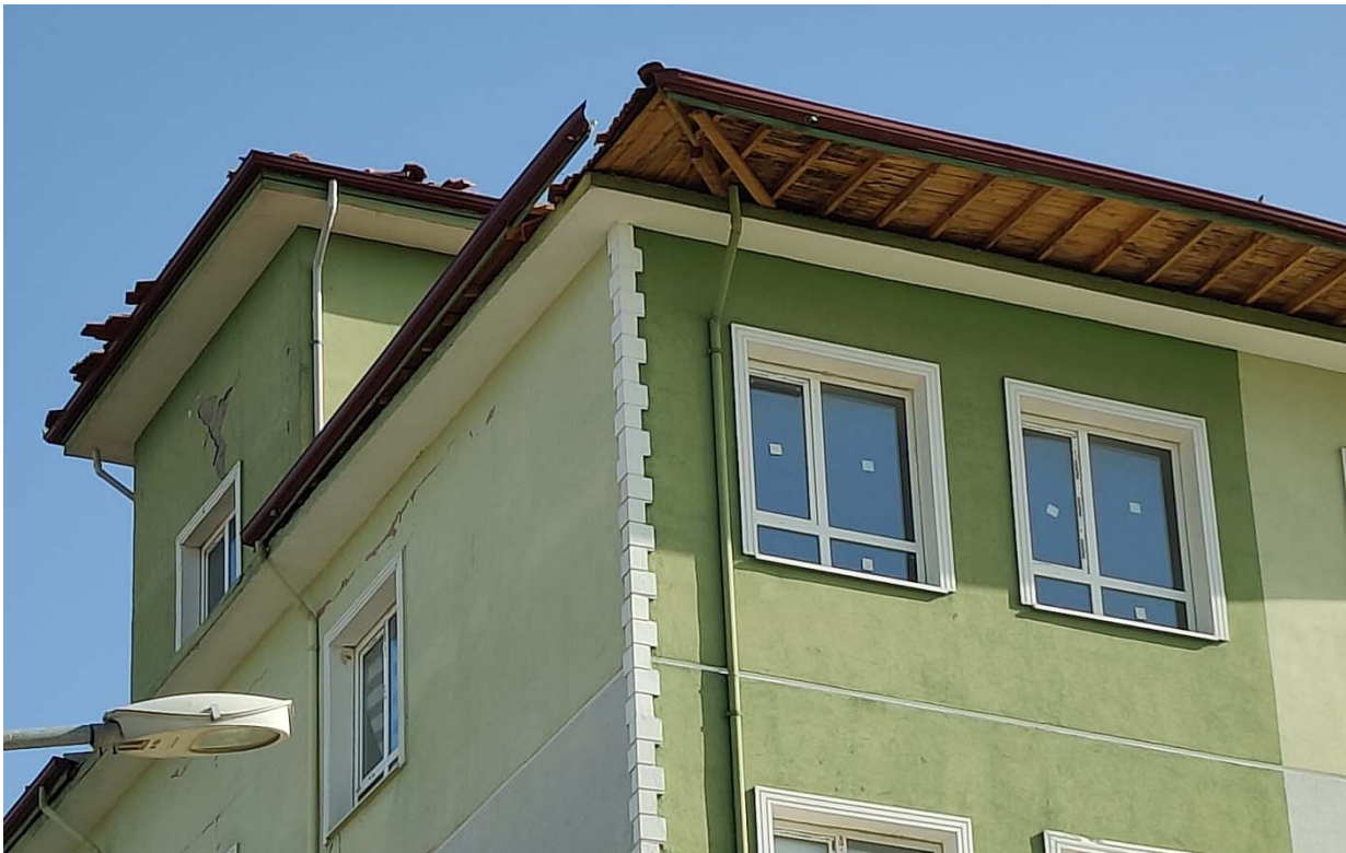
Fig. 7 – Partial collapse of the roof cover.
