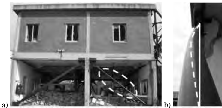
Figure 19. Damage pattern: -0.2% of interstorey drift ratio.
