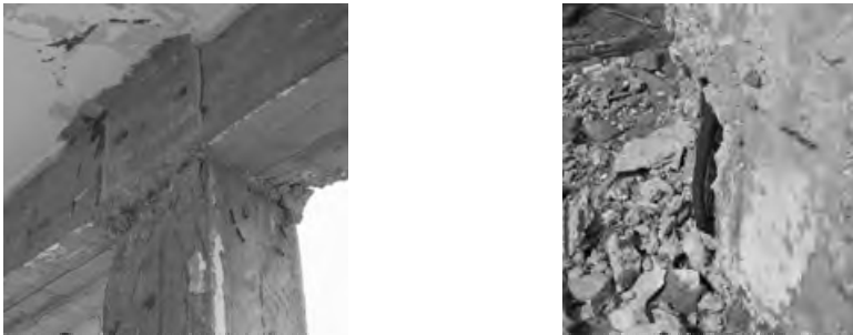
Figure 6. Damages in the column due to the execution of the experimental test with SMA bracings in the transversal direction of the building.
