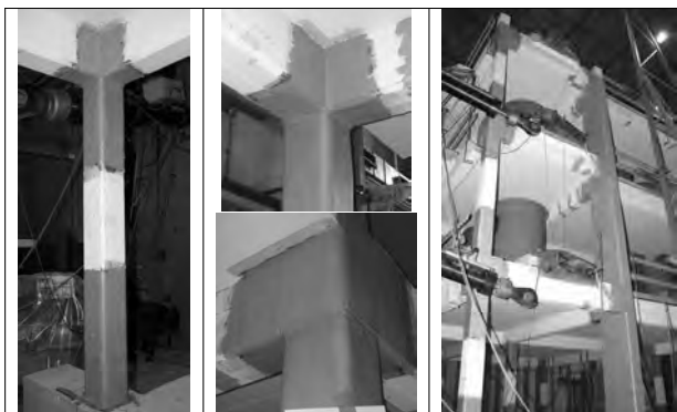
Figure 30. Column confinement and shear strength of corner joints (a); shear strength of wall-type column and retrofitted structure overview (b).
