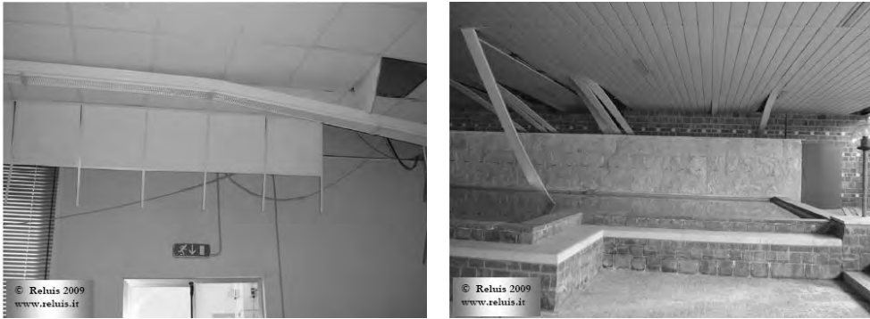
Figure 7. Failure of ceiling panels.
