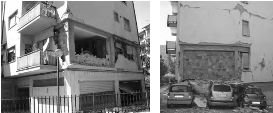
Figure 4. Example of damage to masonry infills in RC multi-storey buildings.
