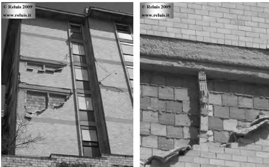
Figure 6. Damage to masonry infills in RC multi-storey framed buildings.
