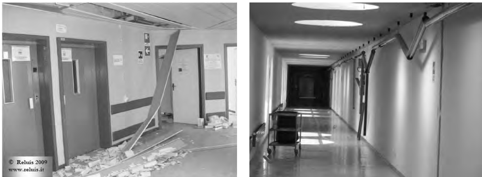
Figure 8. Damage observed in the Saint Salvador Hospital, L'Aquila.
