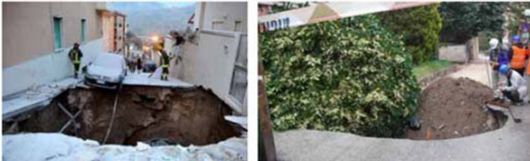
Figure 62. Sinkholes in L'Aquila.
