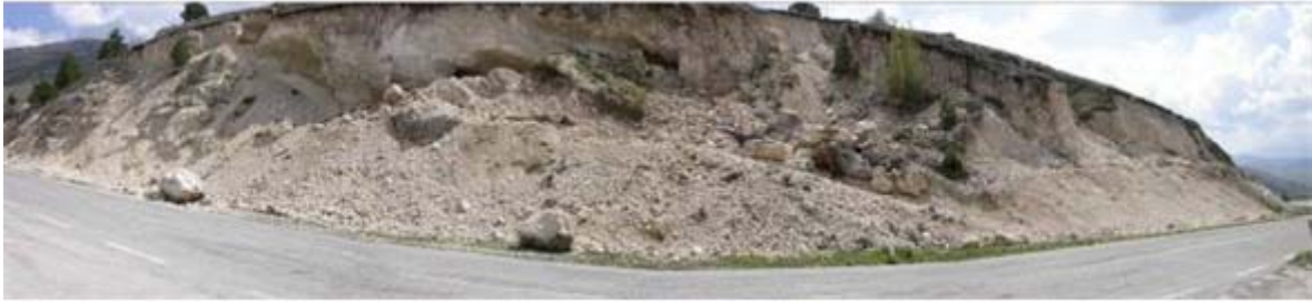
Figure 59. Slump along the road from Barisciano to S. Stefano (Photo by D. Calcaterra and M. Ramondini, University of Naples).
