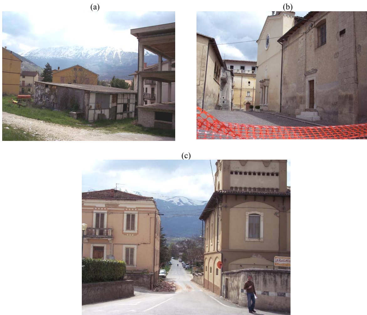
Figure 47. Monticchio : (a) D0 damage level on different building structures; (b) D0 damage on monumental masonry buildings; (c) D1 damage (fall of the cornice) on a masonry building.
