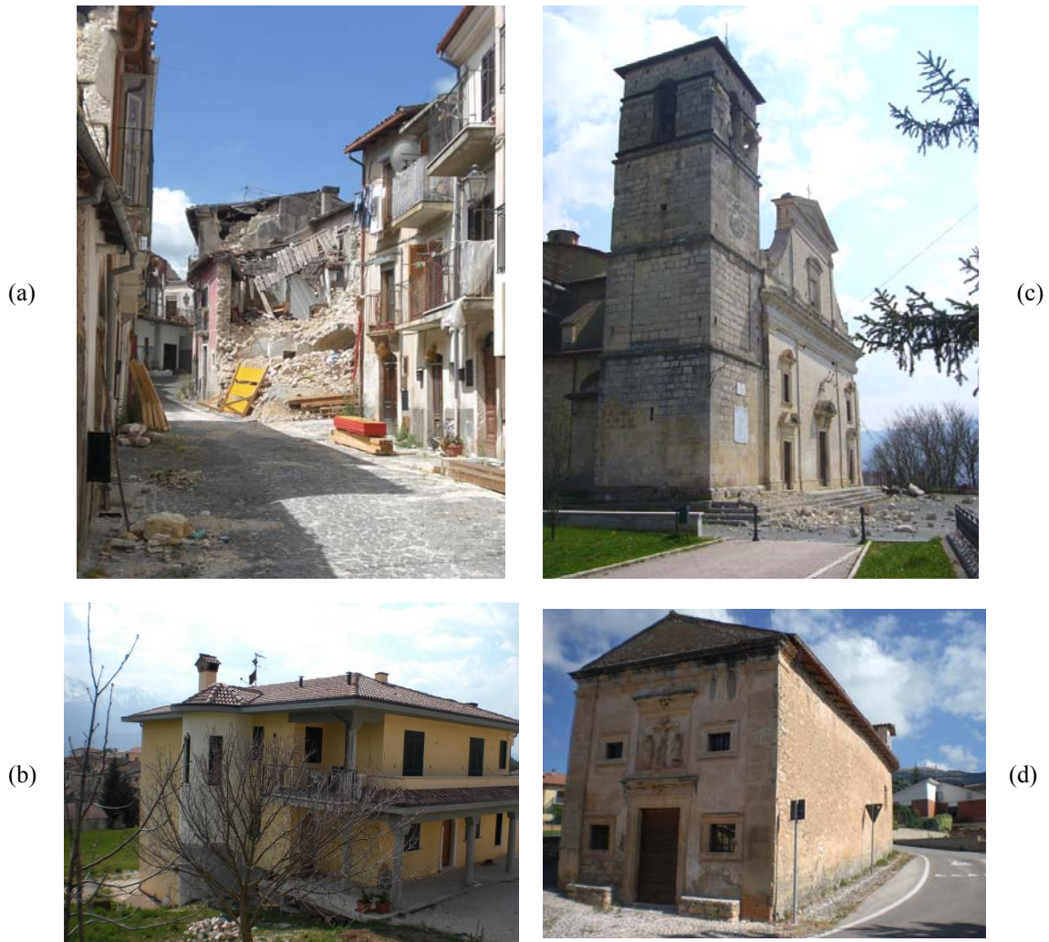
Figure 54.. Poggio Picenze: (a) variable damage (D3-D4) on masonry buildings of different style, (b) undamaged r.c. house (D0) close to the (c) monumental church (D3); (d) D1 damage in a church built on coarse-grained Pleistocene formation.
