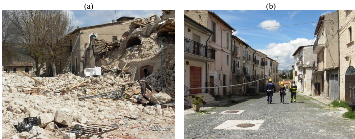
Figure 50. Castelnuovo: (a) collapse (D5) of old masonry buildings on the hilltop; (b) limited damage (D1-D2) to masonry buildings at the toe of the hill.
