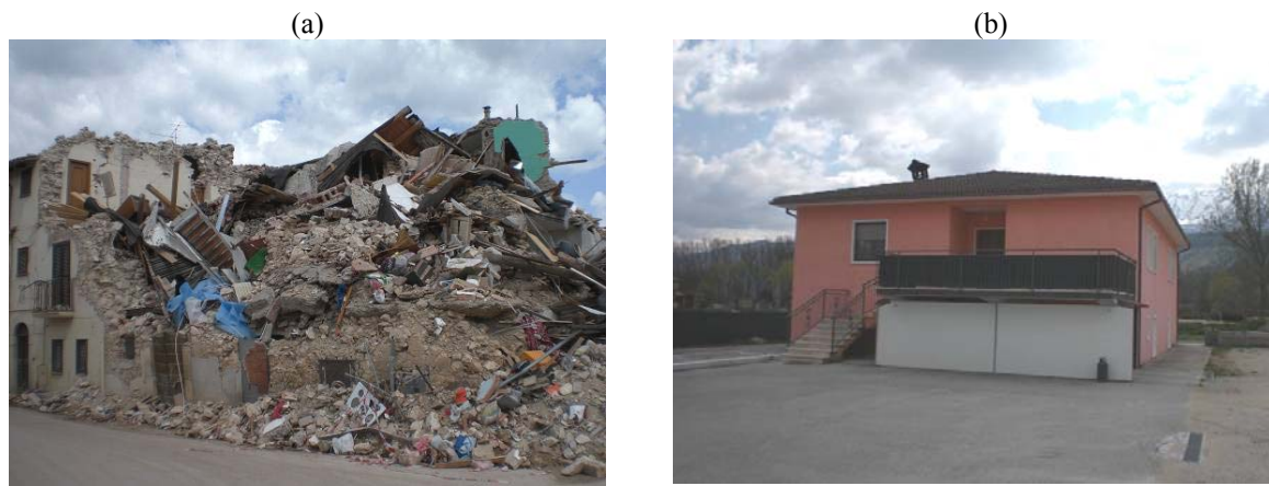
Fig. 46. Onna: (a) D5 damage level on masonry building structures; (b) D0 damage on a r.c. building (except for the tilting of the chimney).
