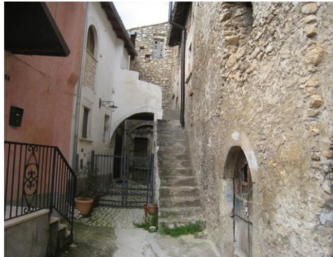
Figure 51. Typical unreinforced masonry structures in the village of San Pio delle Camere suffered no damage (D0), or slight cracking (D1). Structures in this village are similar to those in Castelnuovo.
