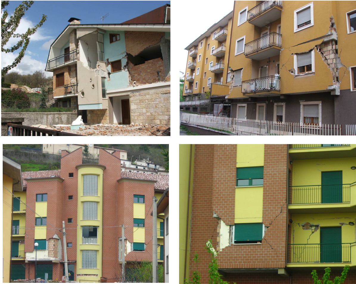
Figure 1 – Collapse of non-structural components in residential reinforced concrete (RC) multi-storey framed buildings in the outskirts of L’Aquila during the 6 April 2009 (Italy) earthquake, designed according to allowable-stress ( top ), limit state ( bottom ) seismic codes .
