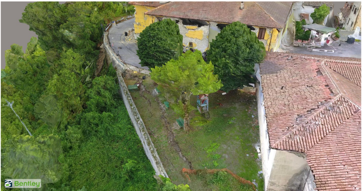
Figure 4.42. Model image of a rotated retaining wall (3.5-degrees) and the subsequent soil graben behind the wall (42.69446 N 13.24980 E).
