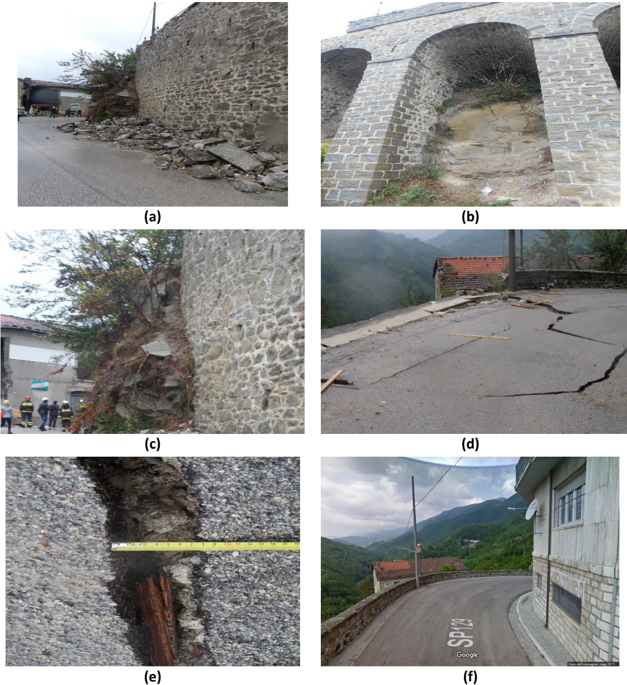
Figure 7.4. Masonry retaining wall in Arquata del Tronto (42.771898N, 13.296715E): (a) partial collapse of the wall parapet, (b) arch masonry structure, (c) marl blocks along the SP129 road, (d) road instability at the top of the wall, (e) opening of the cracks developing along the direction parallel to the road axis, (f) Google Earth view of the site (dated May 2011).
