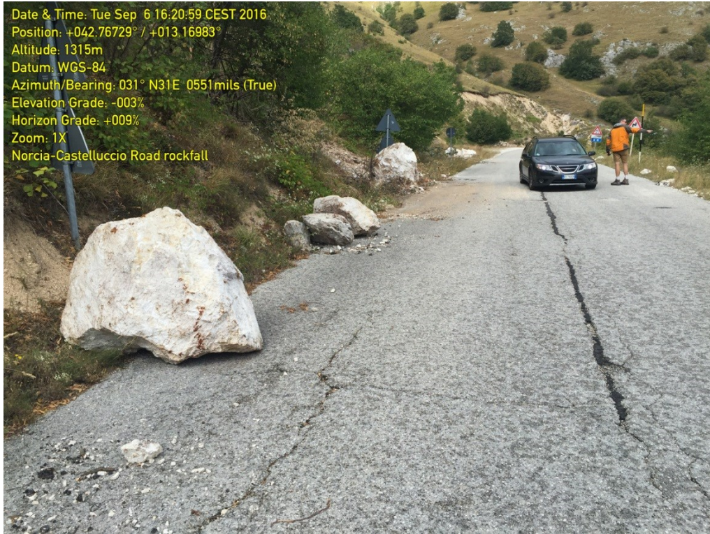
Figure 4.18. Example of rock fall below the Plano Grande on SP477. Blocks as large as 3 to 4 m across came to rest on the flat roadbed below a prominent outcrop of limestone (42.76729 N 13.16983 E).
