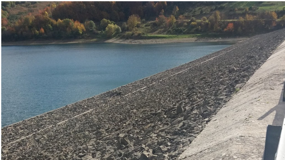
Figure 7.15. Poggio Cancelli embankment dam on the Campotosto reservoir (L'Aquila): photo of the upstream face taken on October 19, 2016 (42.557106°N, 13.338342°E).
