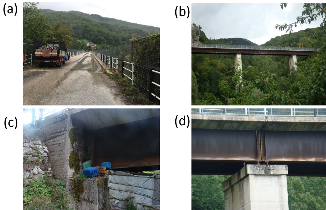
Figure 6.2. Ponte Ramazzotti - Composite steel and concrete bridge along the SP20 in Colle (42.7276 deg, 13.311 deg): overview of the bridge (a,b), abutment (c) and bridge support (d) details.
