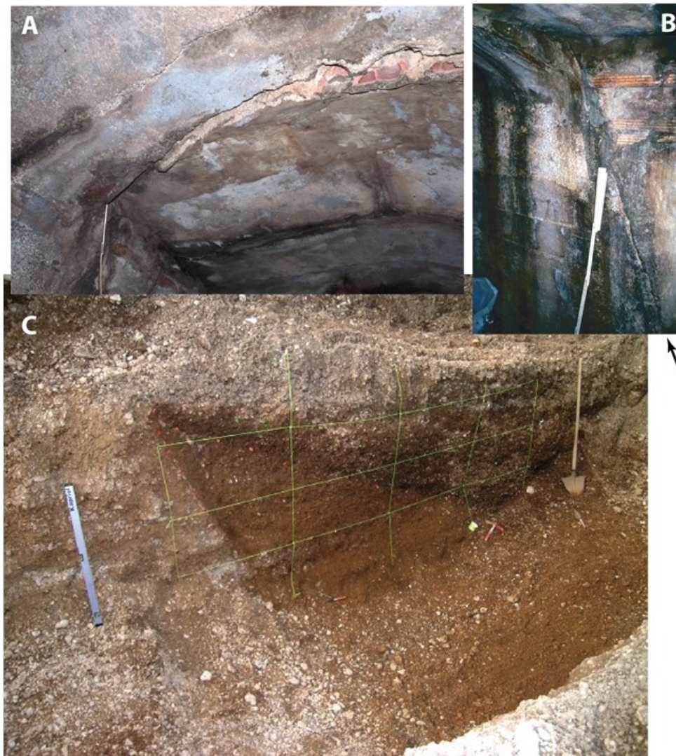
Figure 2.5. Norcia fault: emergence of active fault splays in the settled area of Norcia: a, b) vault and walls of a cellar displaced by a fault which activated during the earthquake of 1979; c) panoramic view of the trenches excavated by Galli et al. (2005) in the suburbs of Norcia: the fault places Middle Pleistocene alluvial gravels in contact with colluvial units ranging in age from the Upper Pleistocene (i.e. the lowermost unit with the orange matrix in the hanging wall) to the 18th century AD.
