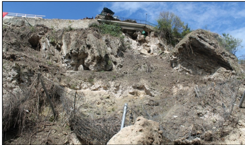
Figure 5.30. Landslide affecting the southern portion of Pescara del Tronto.
