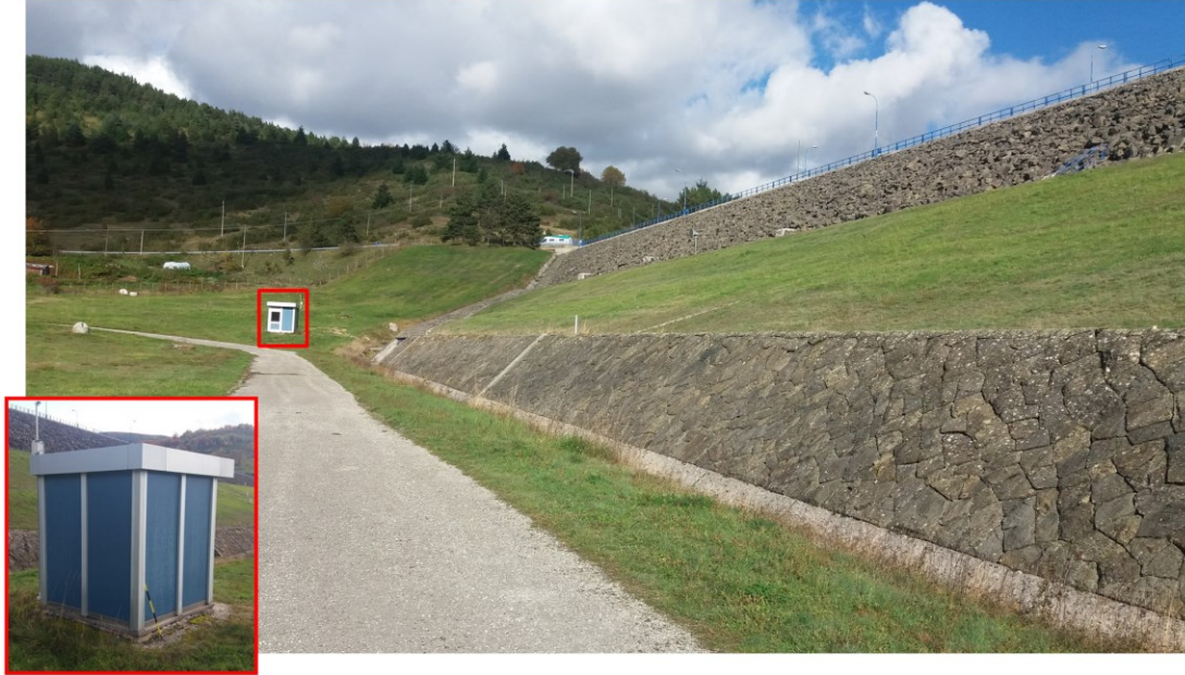
Figure 7.17. Downstream face of the Poggio Cancelli dam (October 19, 2016) with a close-up view of the light blue box hosting the PCB station (42.558022°N, 13.337990°E), which, during the August 24 earthquake, recorded a peak ground acceleration of about 0.31 g.
