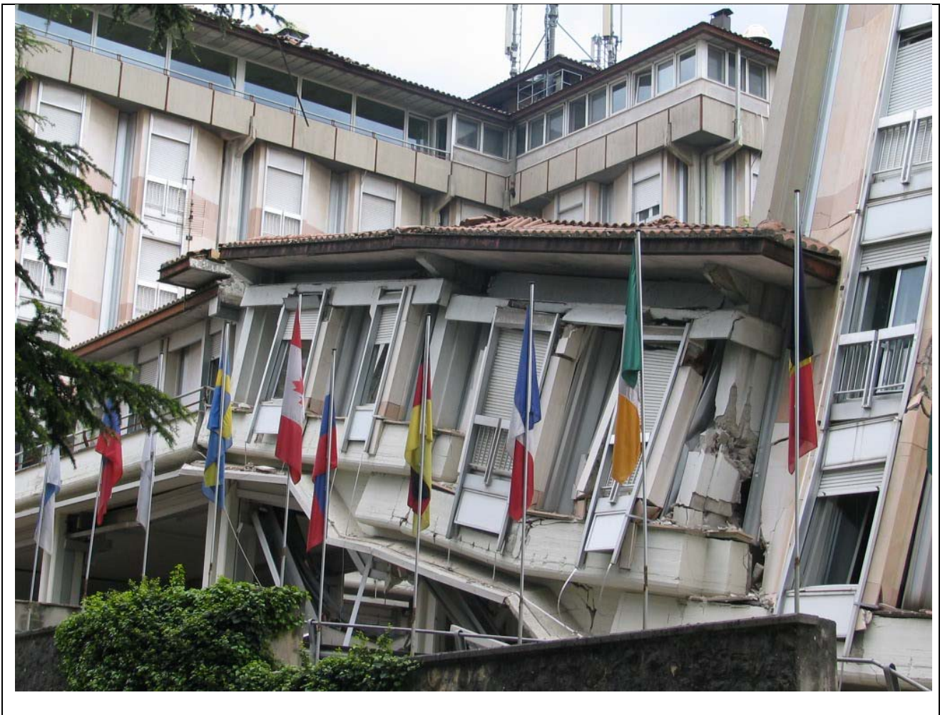
Reinforced concrete building in L'Aquila - via Giovanni XXIII (Hotel Duca degli Abruzzi)
