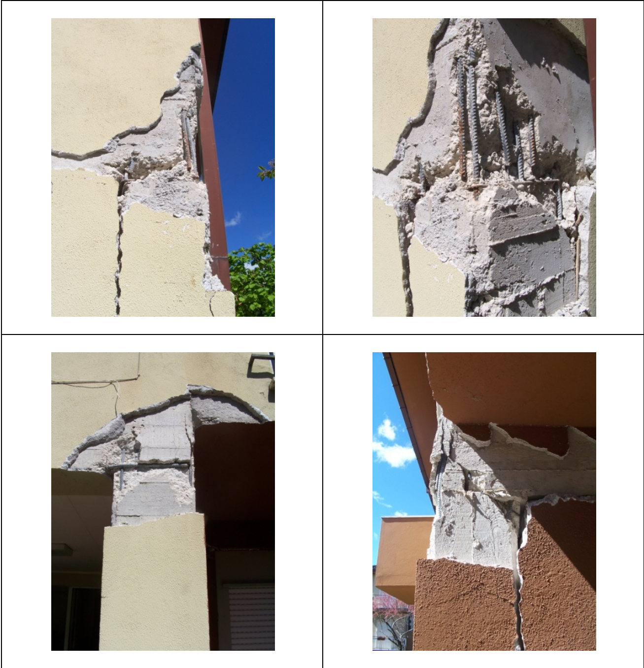
Reinforced concrete building in Paganica - via San Vincenzo, 9 Photo by Bursi, Dusatti and Pucinotti
